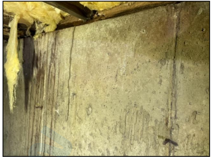
Settlement cracks noted
