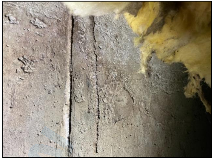
Termite shelter tubes
