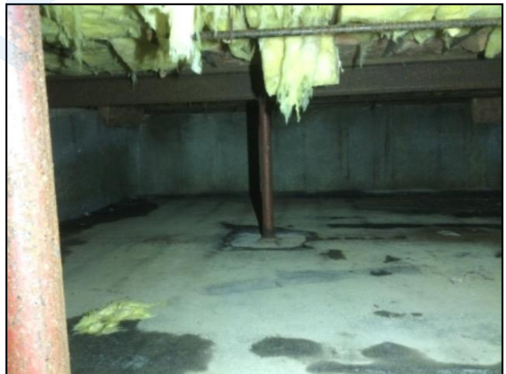
Fallen insulation in the floor structure
