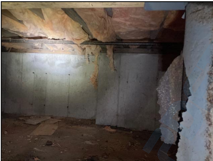
Settlement cracks noted
