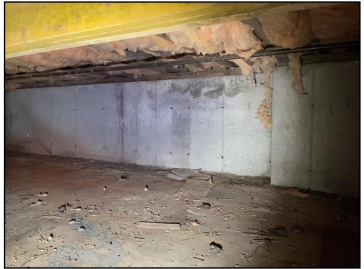
Settlement cracks noted
