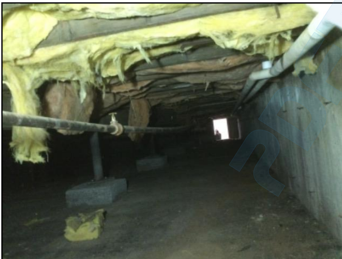
Fallen insulation in the floor structure
