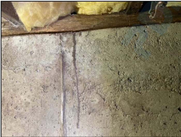
Termite shelter tubes
