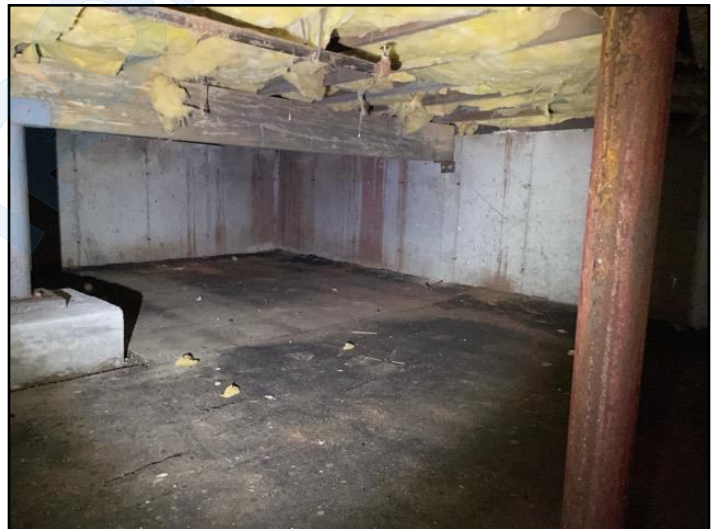
Settlement cracks noted
