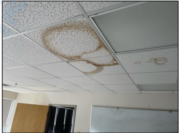
Numerous signs of leaks
