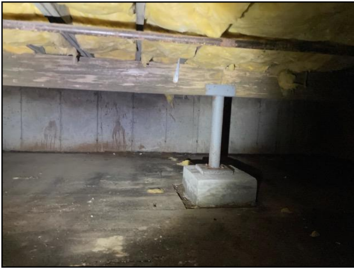
Settlement cracks noted
