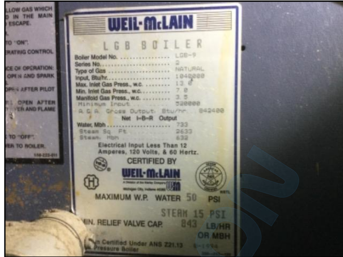
Forced hot water boiler in basement
